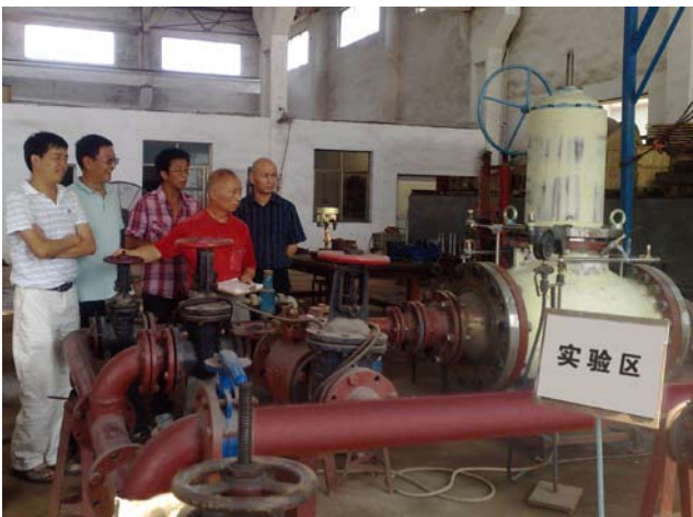
构皮滩电站工作人员在我生产基地进行产品验收试验 Staff from Goupitan Power Station is carrying out inspection acceptance of products at our manufacture base
